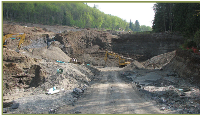
Significant earthworks can compromise natural slope conditions and neighbourhood character.
