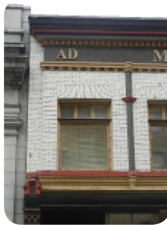
Photo 32 - Historic building incorporates cornice treatments along the roof line and across the façade
