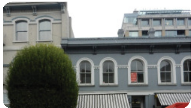
Photo 30 - Roof line variation between adjacent buildings
